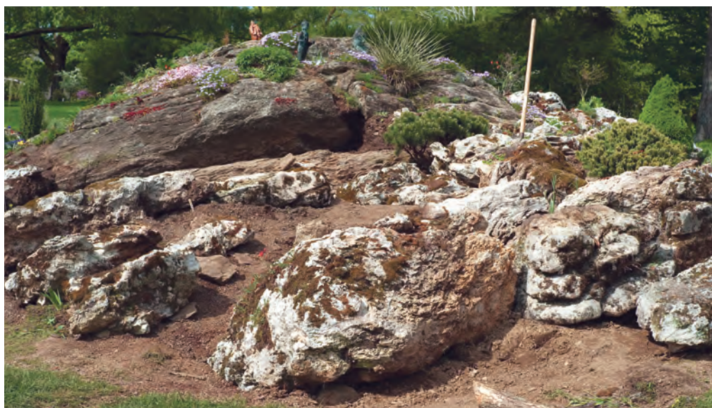
The excavated ledge at the back with some rocks laid in front
